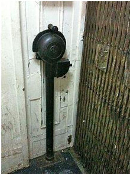
Otis 1920s controller, operational in a New York City apartment building
