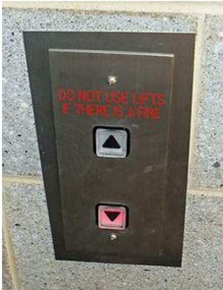
An external control panel
