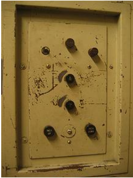
Manual pushbutton elevator controls
